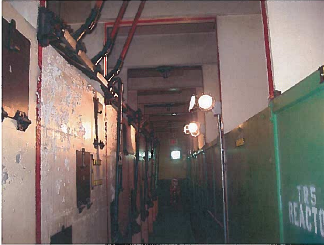
Room with Gang operated disconnects and 4.16kV bus – Black doors on left wall provide access to each phase energized bus. 1 of 2 such rooms
