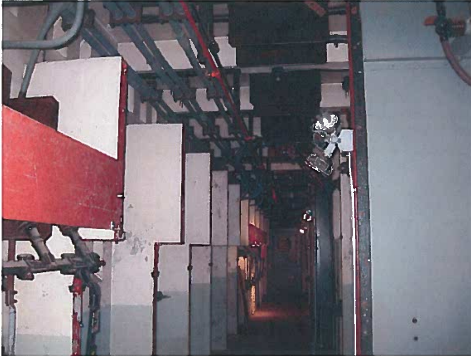
Room with 4.16kV -4 switches (left), -3 disconnects (ceiling)
