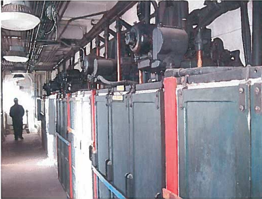
One of 7 Breaker Rooms with H-Type Breakers
